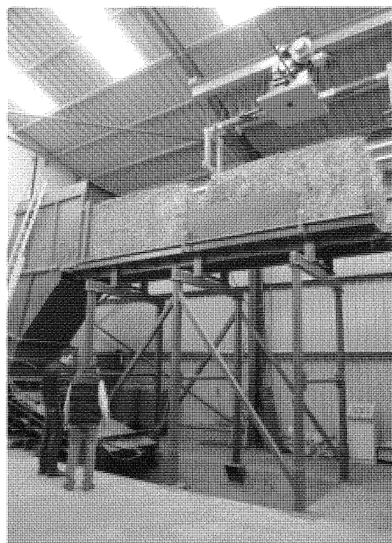
Oil seed rape straw bales being loaded into boiler
