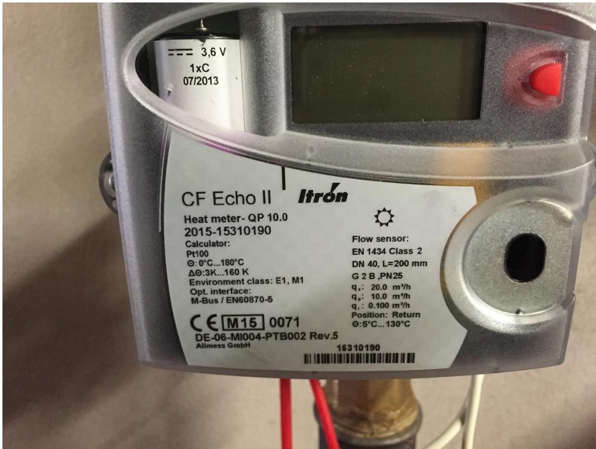
Boiler 4 Heat meter HMrhi
