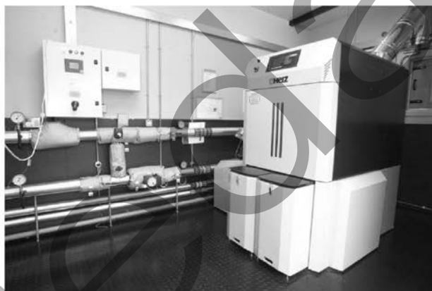
Herz 99kW inside a container unit.
